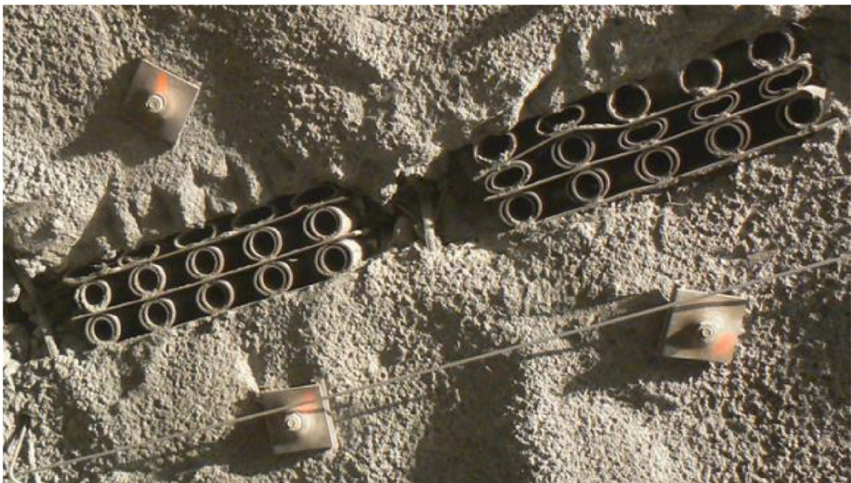
Fig. 2: Grid girder rigid support with compression elements [Bochumer Eisenhütte GmbH & Co. KG]
